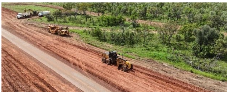
Carpentaria Highway upgrade –construct stage 2 ch 50 – 140 km (earthworks between ch 63 – 68 km) Photo extracted from the February 2024 Project Report compiled by Exact Contracting
