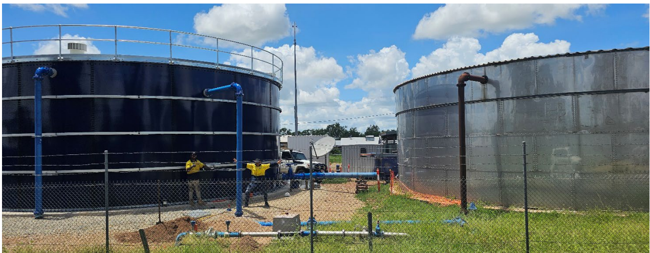
Beswick and Jilkminggan - new ground level tanks (Beswick). Photo courtesy of Power Water Corporation.
