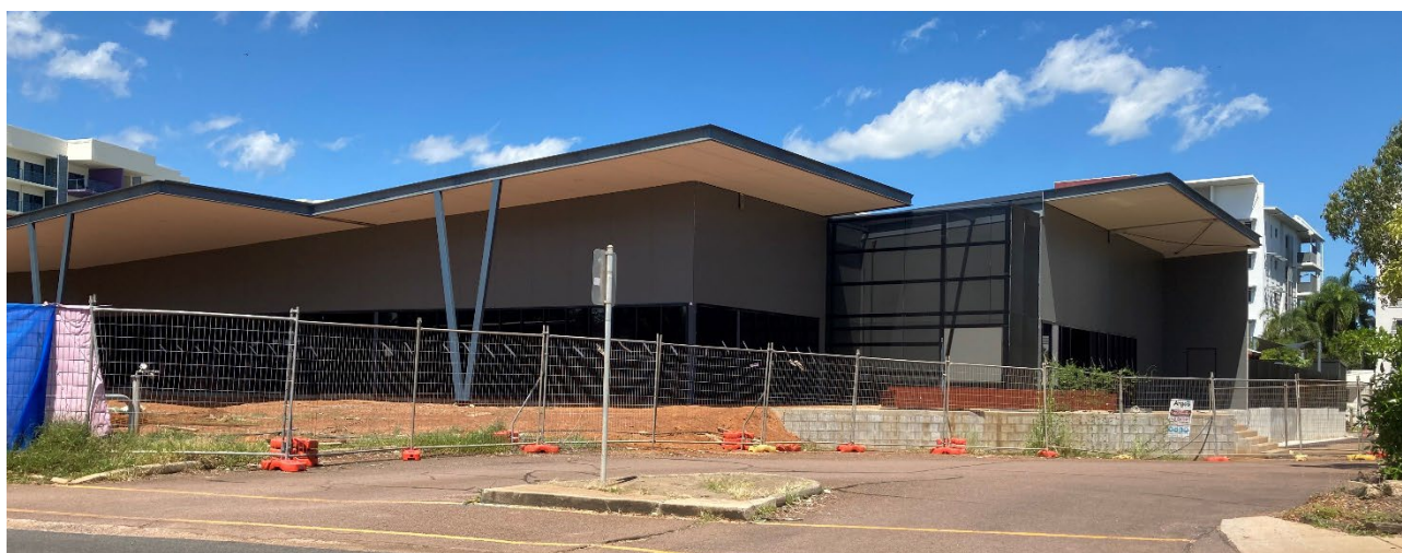
Nightcliff - 69 Progress Drive - redevelopment - childcare centre, community centre, offices and food premises-café
