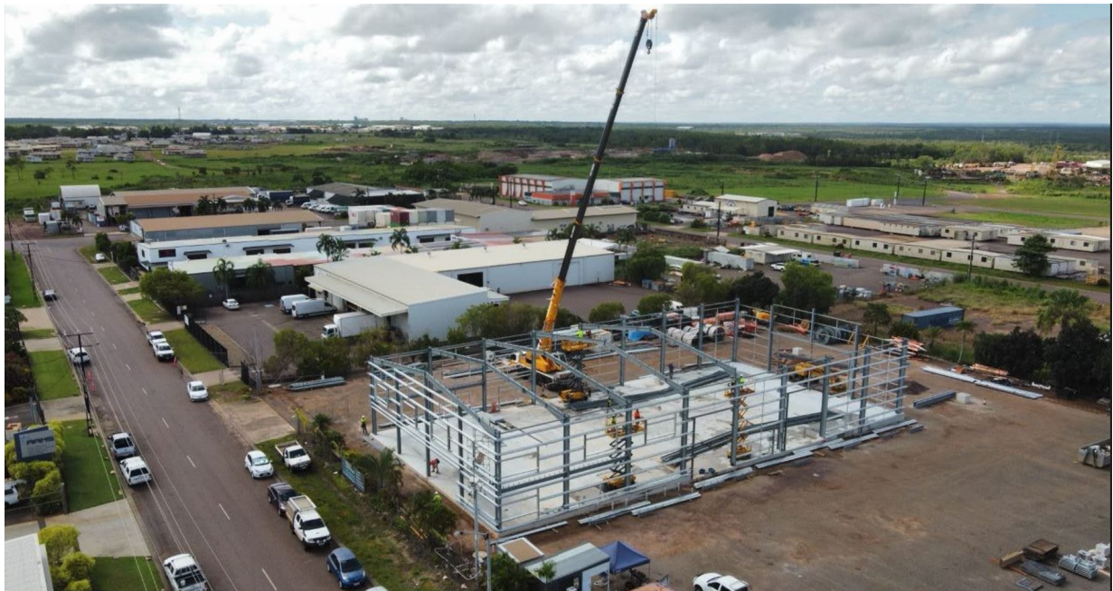
Berrimah - 14 Anictomatis Street - MEC warehouse and office Image courtesy of Molloy Electrical Contracting Pty Ltd and DC Ideas Pty Ltd
