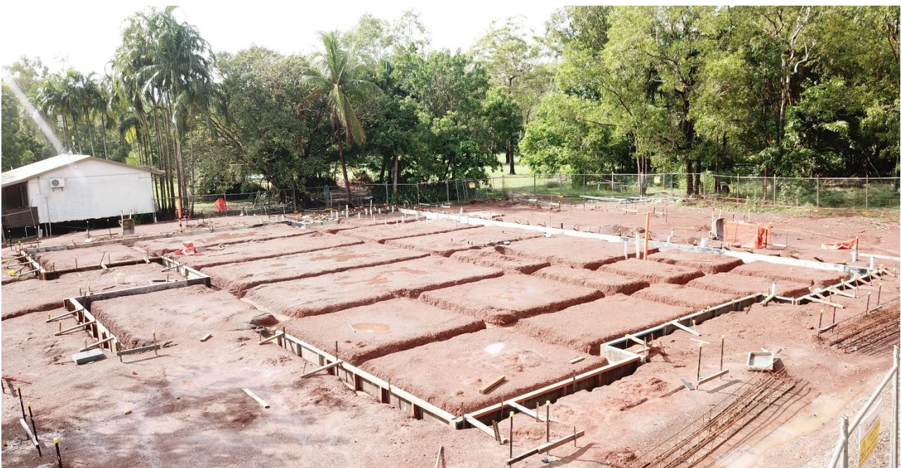
Bees Creek - National Critical Care and Trauma Response Centre (NCCTRC) - training facility Preliminary concepts credit to Mode Designs
