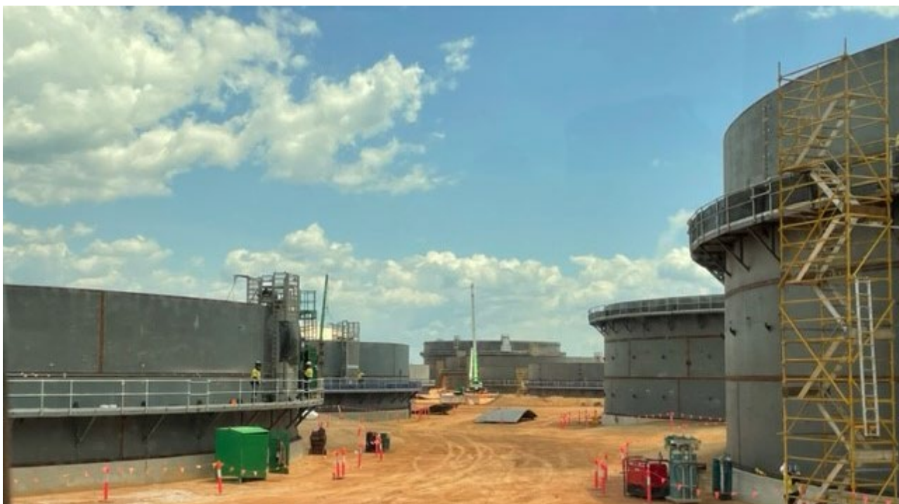
East Arm - Bulk Liquids Area - Crowley Project Caymus - construct U.S Defence jet fuel storage facility
