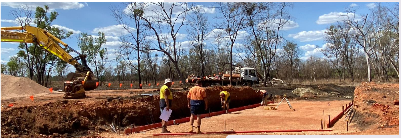
Central Arnhem Road (Bulman package) - upgrade and bitumen seal ch 250.8 - 254.9 km (culvert 7)
