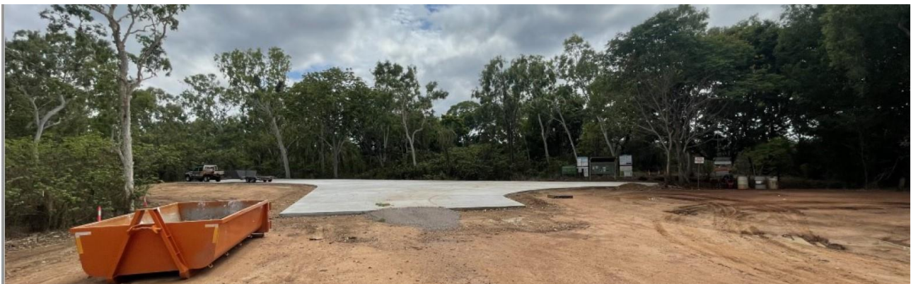
Point Stuart Road - upgrade between ch 69 km to boat ramp turnaround area
