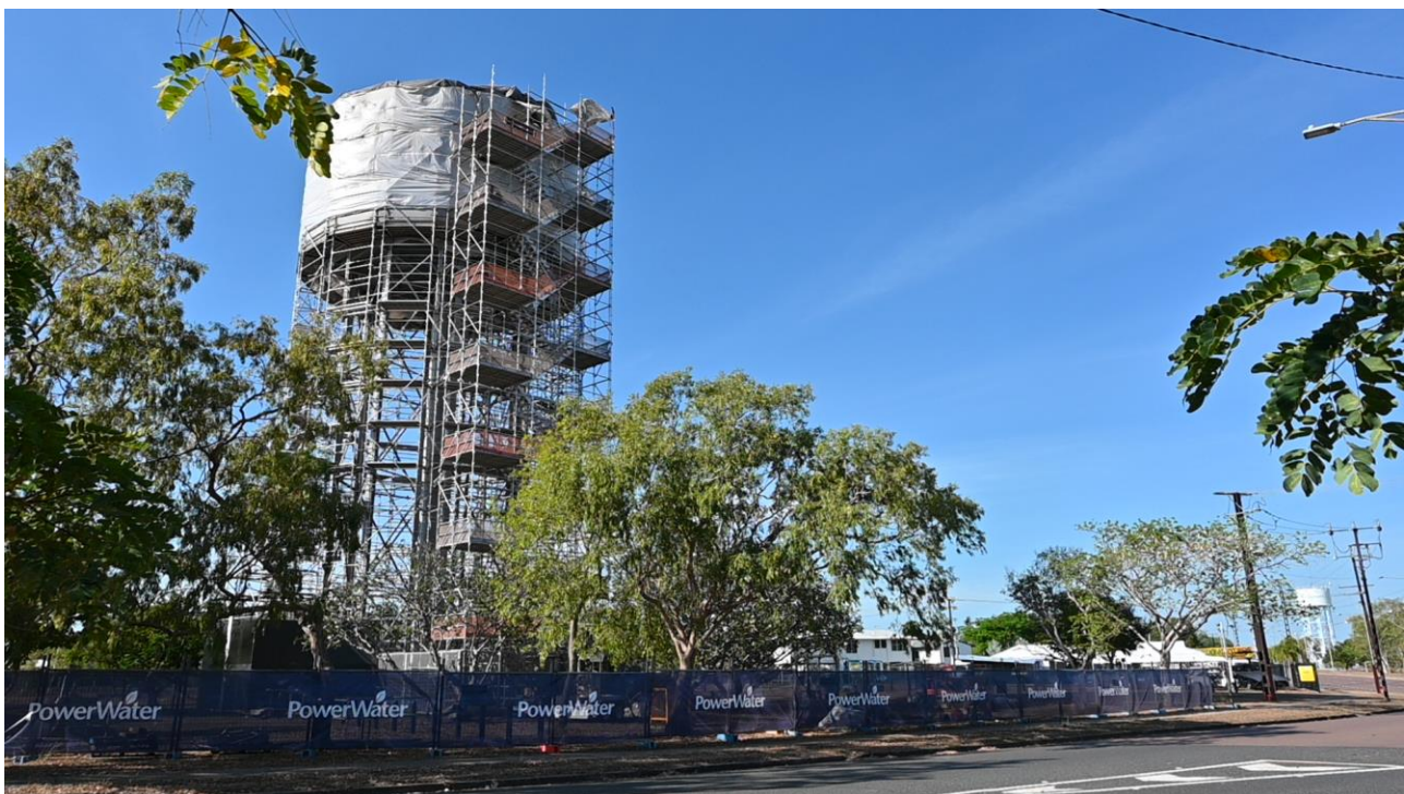
Salonika Elevated Water Tank - roof replacement (Critical Tank) Image courtesy of Power Water Corporation
