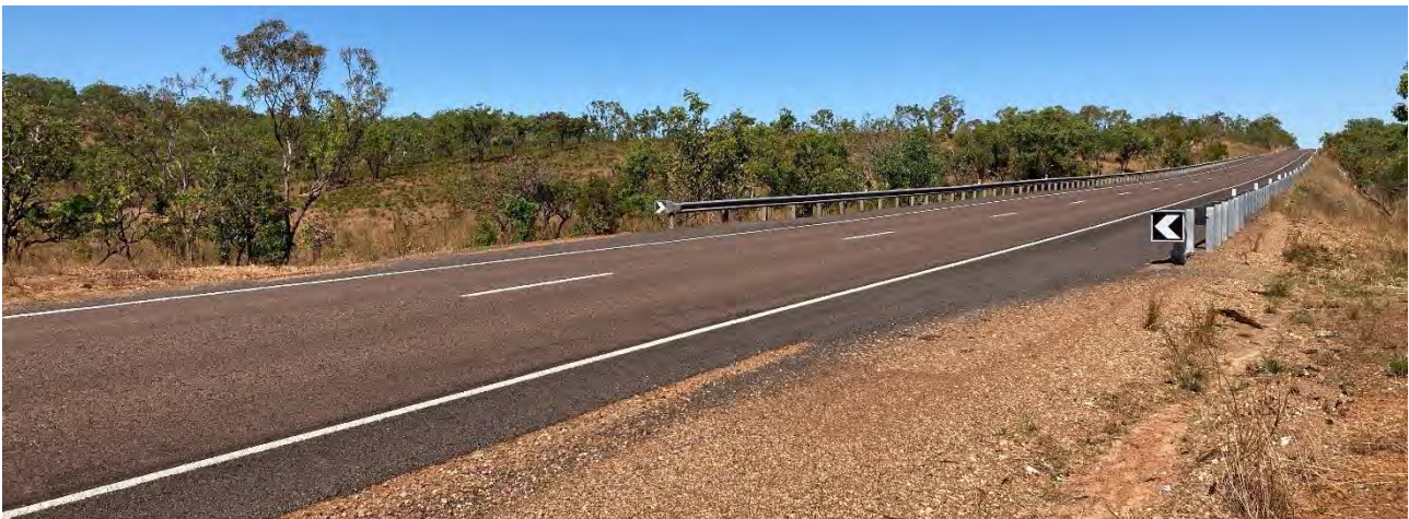
Stuart Highway - shoulder rehabilitation, sealing, safety barrier and culvert extensions from chainage 137 - 165.33 km
