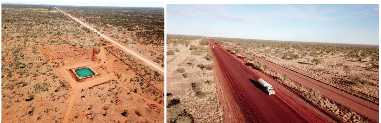
Construction photos: Outback Way – Plenty Highway upgrade to seal chainage 167.11 - 170.15 km and 209 - 224 km
