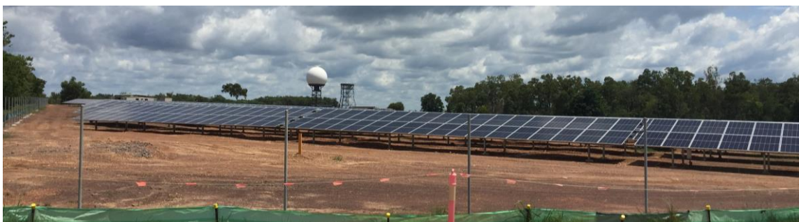
Photo: RAAF Base Darwin and Robertson Barracks - solar photovoltaic power generation systems
