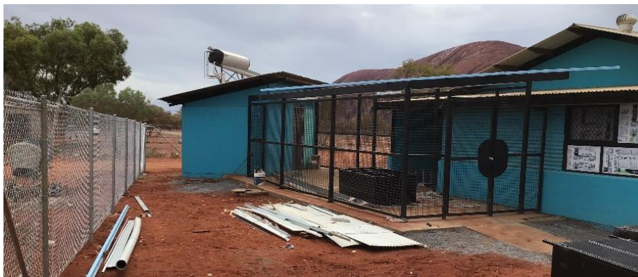
Construction photo: Mutitjulu - NPRH - demolition of 2 dwellings, construction of 2 by 3 bedroom dwellings, and upgrade 26 dwellings
