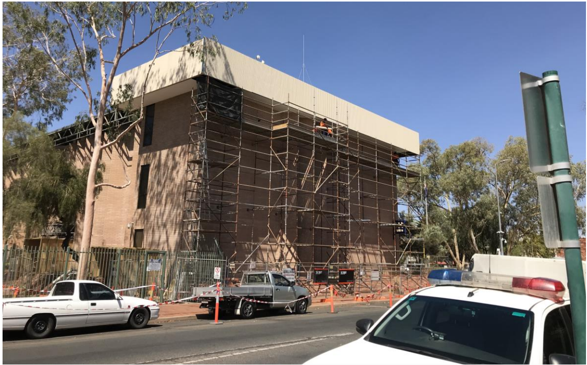
Construction photo: Alice Springs Police Station - remove external linings and replace with new
