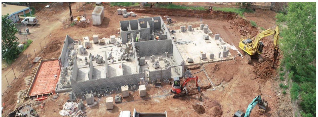
Construction photo: Ngukurr - construction of a new Police Station, houses and Visiting Officer Quarters
