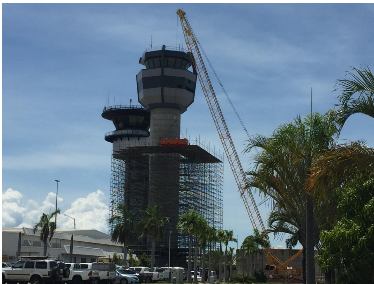
Construction photo (Darwin): RAAF Base Darwin and RAAF Base Tindal- Air 5431 - air traffic control - multi-level facility and sensor equipment building
