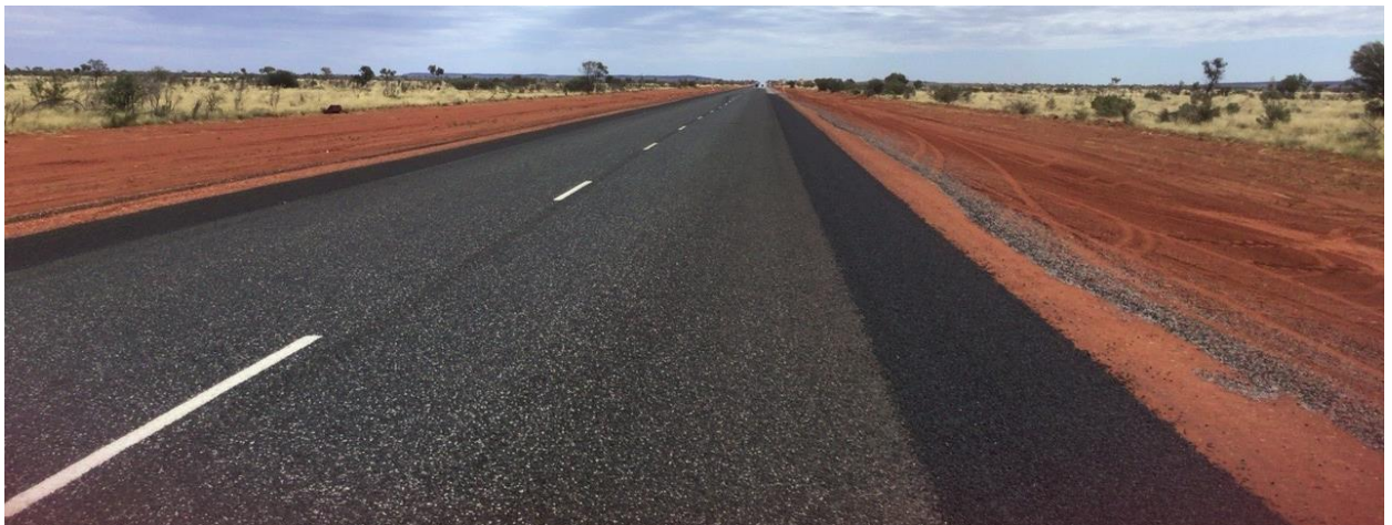
Construction photo: North Stuart Highway - shoulder reconditioning and seal widening works - packages 1 and 2
