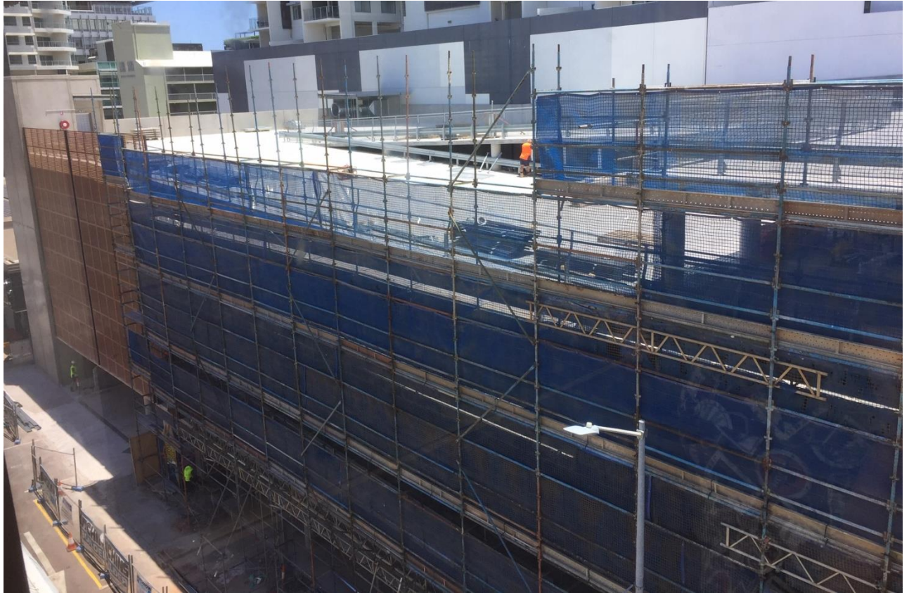
Construction photo: Darwin CBD - 12-14 Litchfield Street - 5 storey public car park building (320 car bays)
