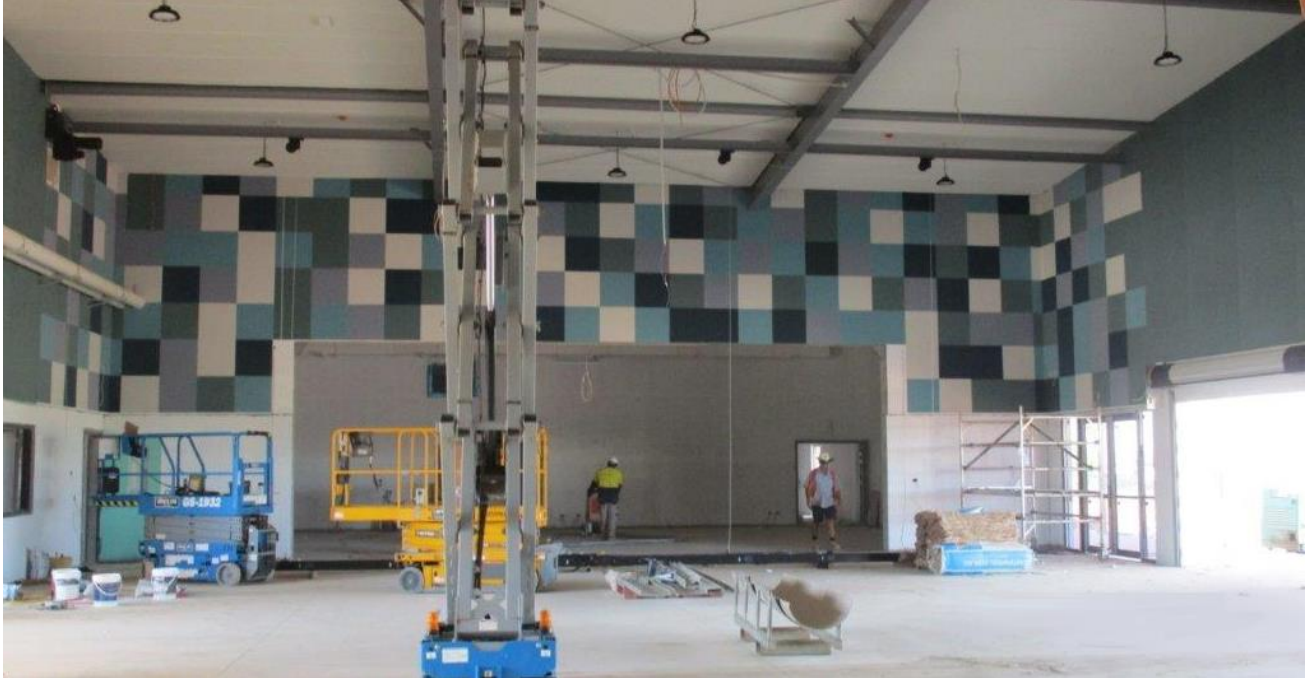
Construction photos: Zuccoli Primary School - stage 2 of the government school and shared facilities
