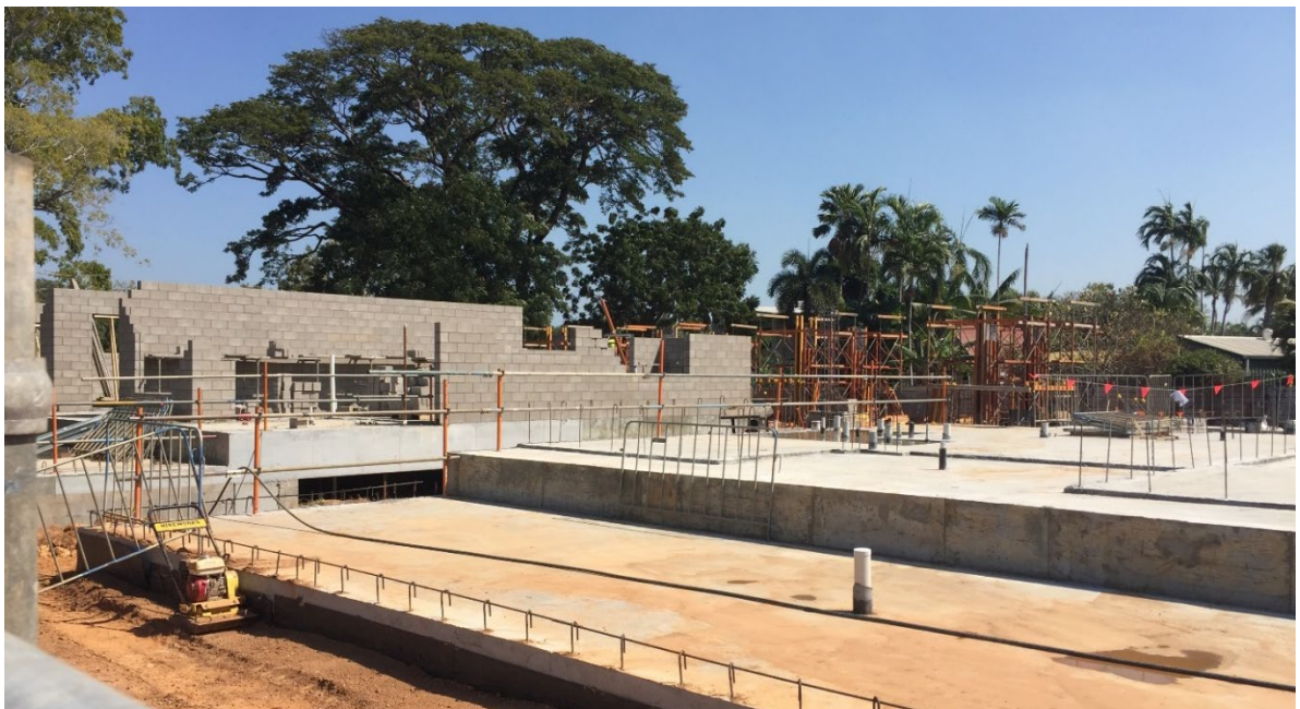
Construction photo: The Narrows - Rubix Apartments - 54 by 2 bedroom multiple dwellings in 5 by 3 storey buildings (in 2 stages)
