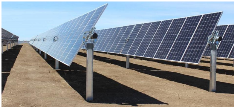
Example of a typical tracking solar array: Yulara Hybrid Power Station - install single axis solar array (6 ha)
