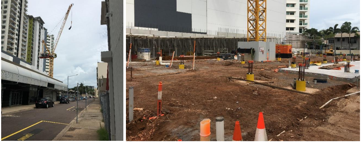
Construction Photos: Darwin CBD - 12-14 Litchfield Street - 5 storey public car park building (320 car bays)
