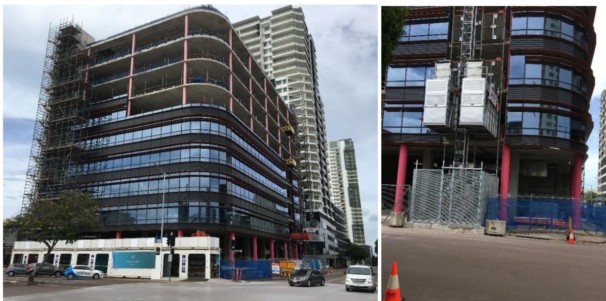
Construction photos: Darwin CBD - 38 Cavenagh Street - Manunda Place development - new 8 storey office building plus 2 levels of basement car parking
