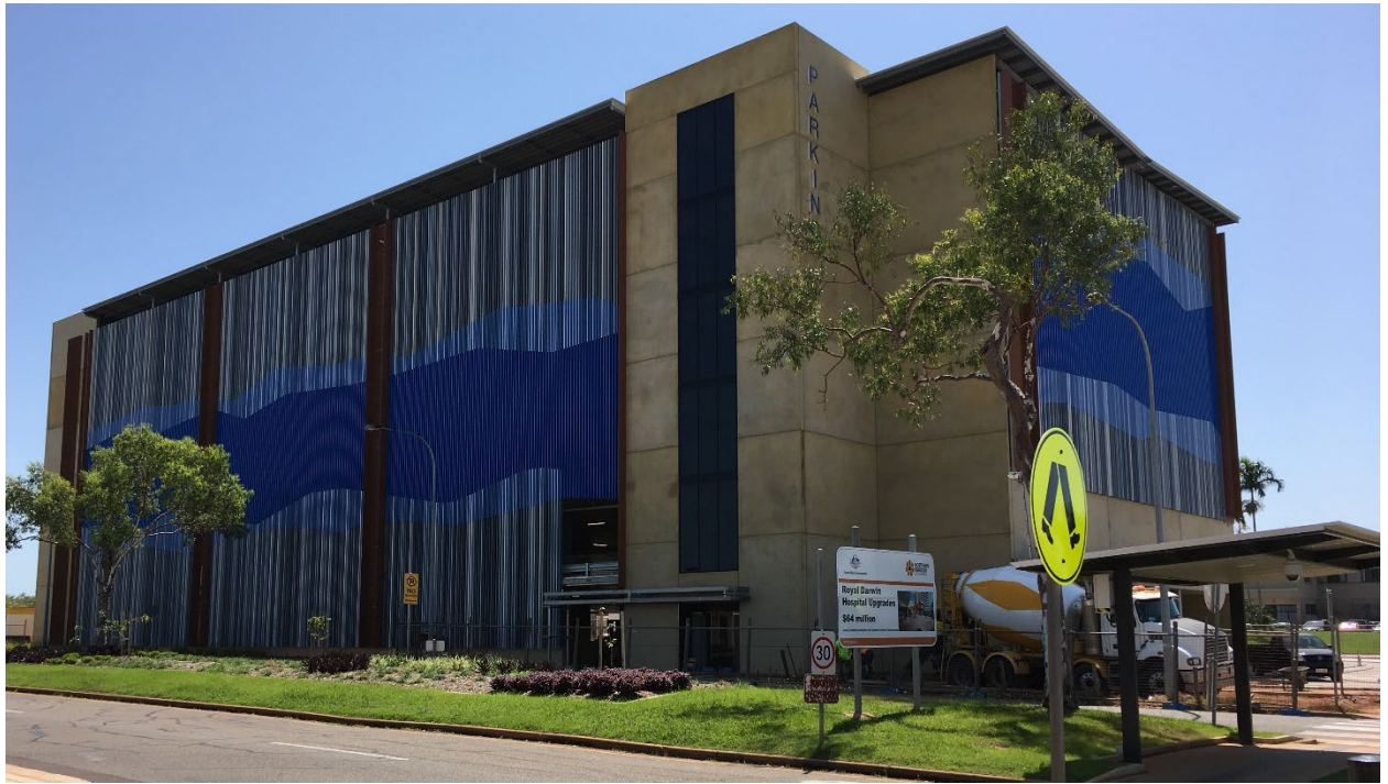
Construction photos: Royal Darwin Hospital - multi-storey car park, increasing on-site car parking
