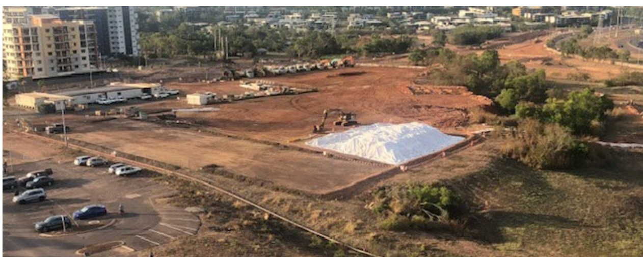
Construction photos: Darwin CBD - Garramilla Boulevard Link - duplication of Tiger Brennan Drive from Dinah Beach to McMinn Street (stage 3)
