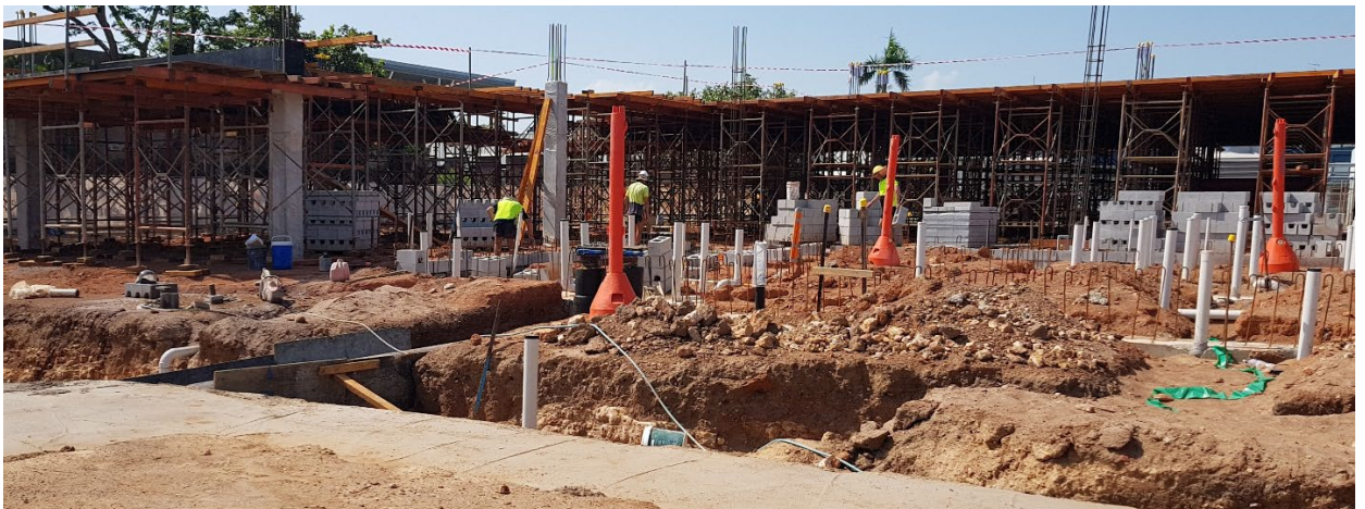
Construction photo: Darwin High School - new Science, Technology, Engineering, the Arts and Mathematics (STEAM)
