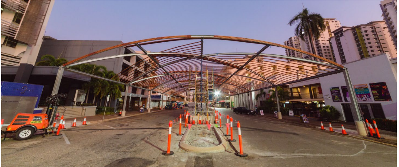
Construction photos: Darwin CBD - Cavenagh Street greening and cooling - new shade structure
