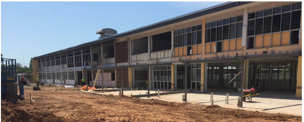
Construction photos: Ludmilla Primary School - Stage 1 Master Plan - refurbish a two storey classroom building to house a new early learning centre, plus an integrated area for a supported play group
