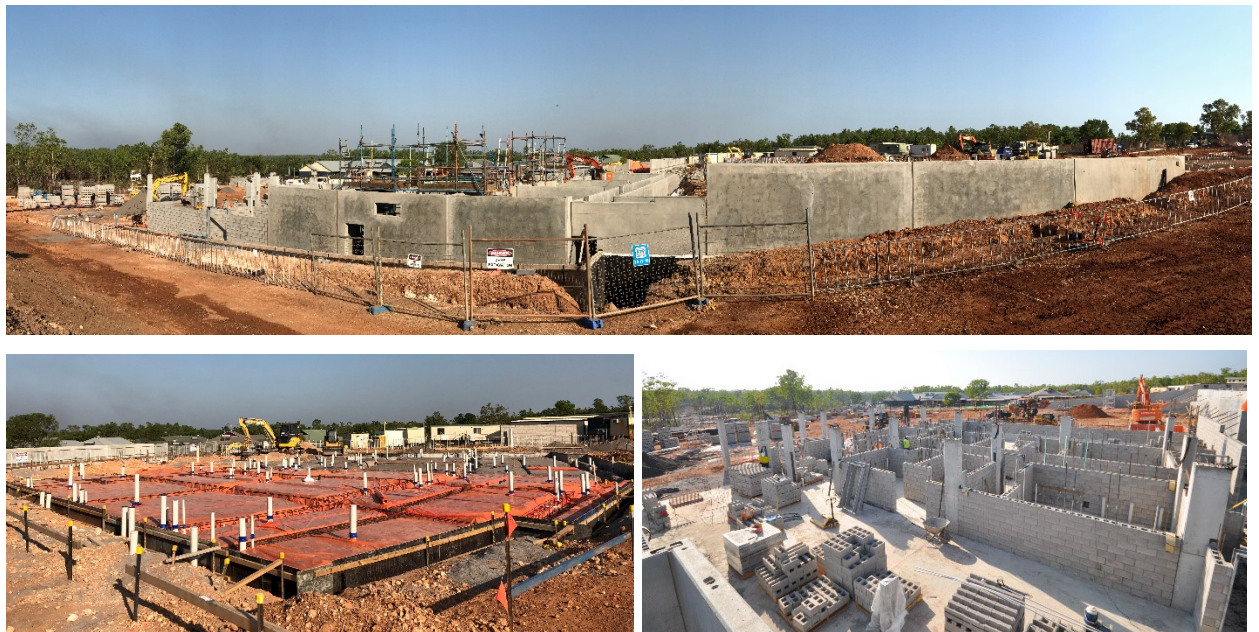
Construction photos: Palmerston Police Station - watch house, emergency operations centre and community hall
