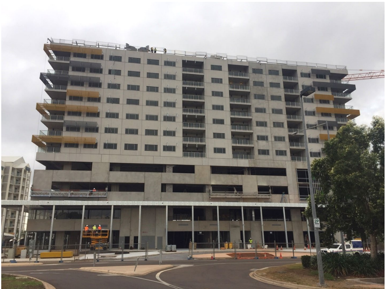
Construction photo: Palmerston CBD - 1 Palmerston Circuit (corner The Boulevard) - 15 storey multiple use development (stage 1)
