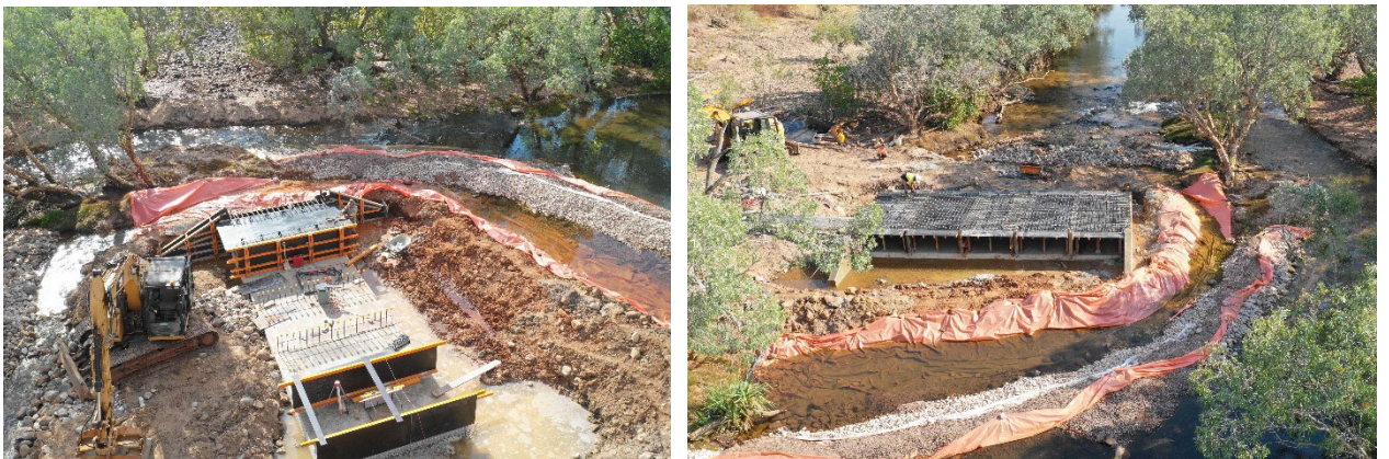
Construction photos: Nitmiluk National Park - stabilisation of 17 Mile Creek crossing to allow vehicle access to Biddlecombe Cascades, to support the development of a new overnight 'glamping' experience
