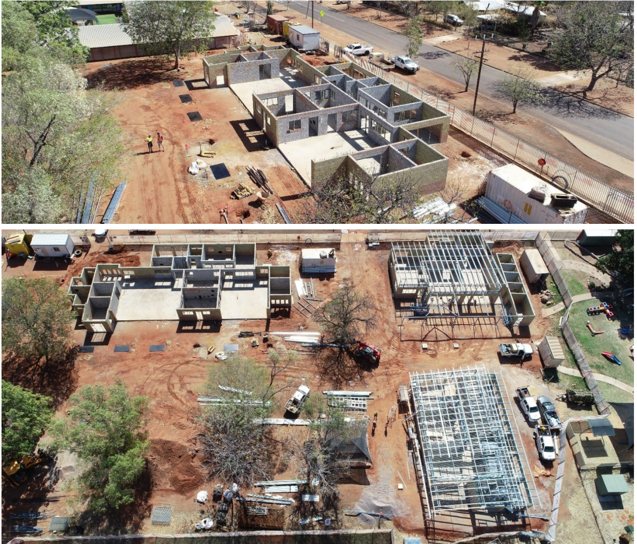
Construction photos: Tennant Creek Early Childhood Integrated Learning Hub - new preschool and child and family centre
