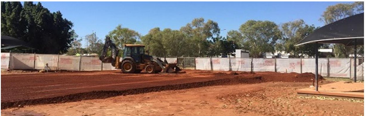
Construction photos and concept: Tennant Creek Early Childhood Integrated Learning Hub - new preschool and child and family centre
