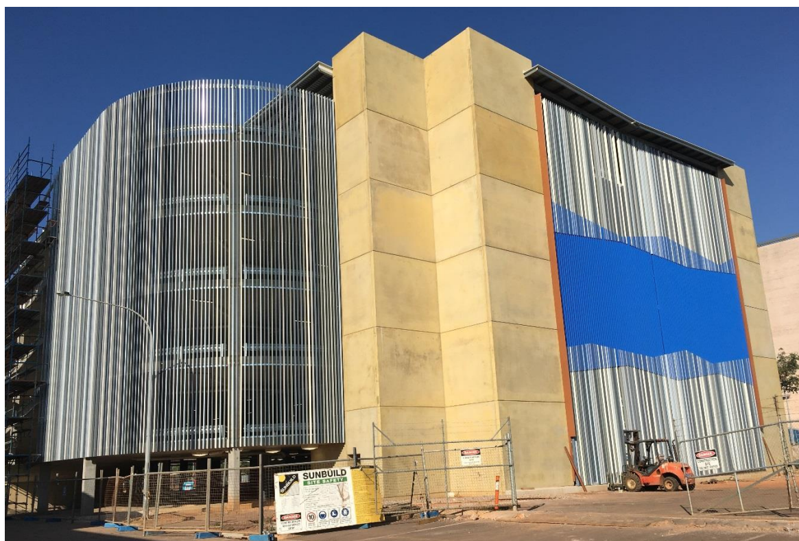
Construction photo: Royal Darwin Hospital - multi-storey car park, increasing on-site car parking
