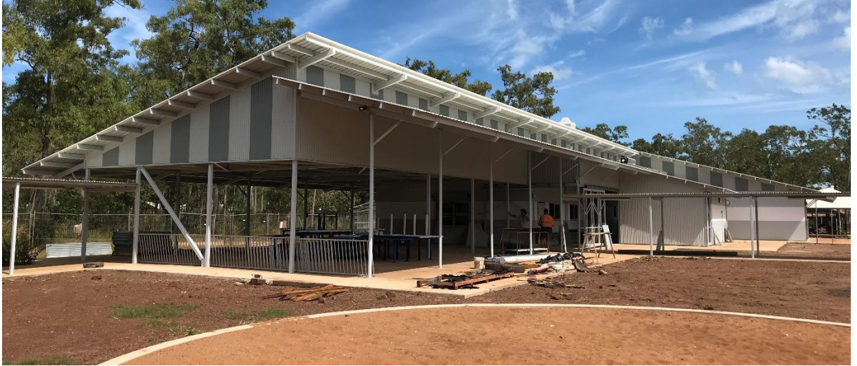
Construction photos: Angurugu School - new school buildings (replace infrastructure destroyed by fire)
