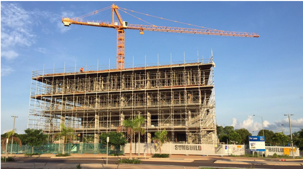
Construction photo: Palmerston CBD - 1 Palmerston Circuit (corner The Boulevard) - 15 storey multiple use development in 3 towers (in 3 stages)
