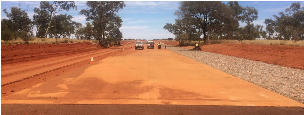
Photo: Tjukururu Road Floodway - upgrade floodways at Armstrong, Irving, Shaw and Chirnside Creeks
