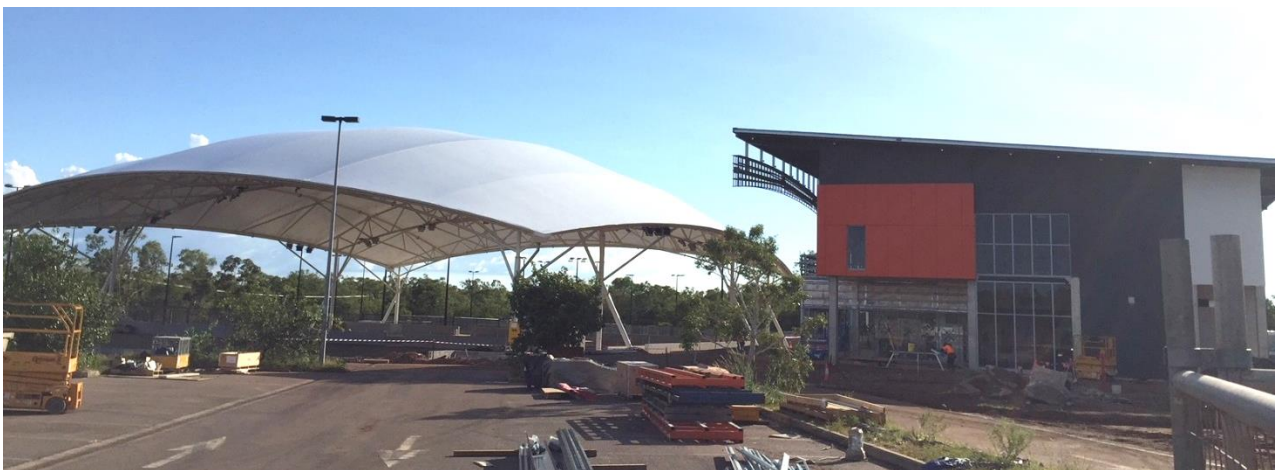
Construction photo: Marrara - new tennis centre including office, restaurant and function centre in a 2 storey building
