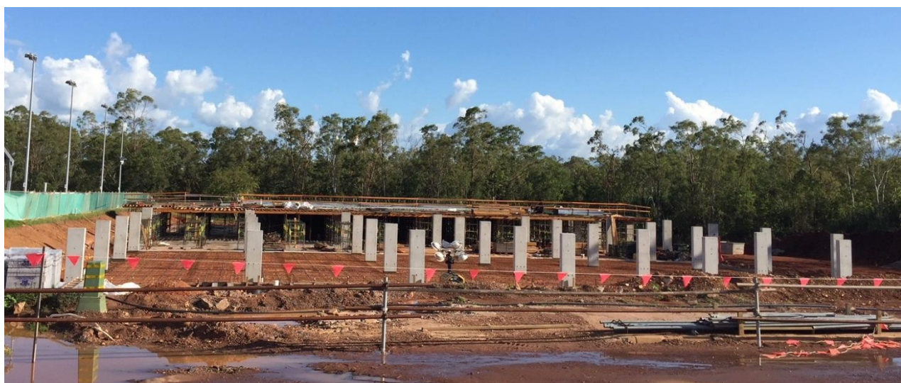
Construction photo: Marrara Sporting Complex - design and construct new indoor netball facility
