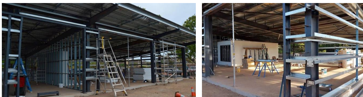
Construction photos: Nhulunbuy - Gove Peninsula Surf Life Saving Club house and function space
