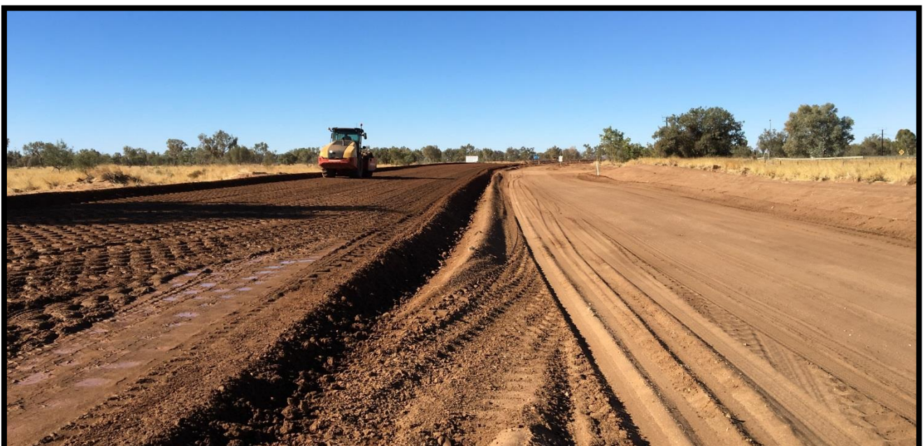
Photo: Plenty Highway - various sections between chainage 245 - 272 km - reform and gravel re-sheet
