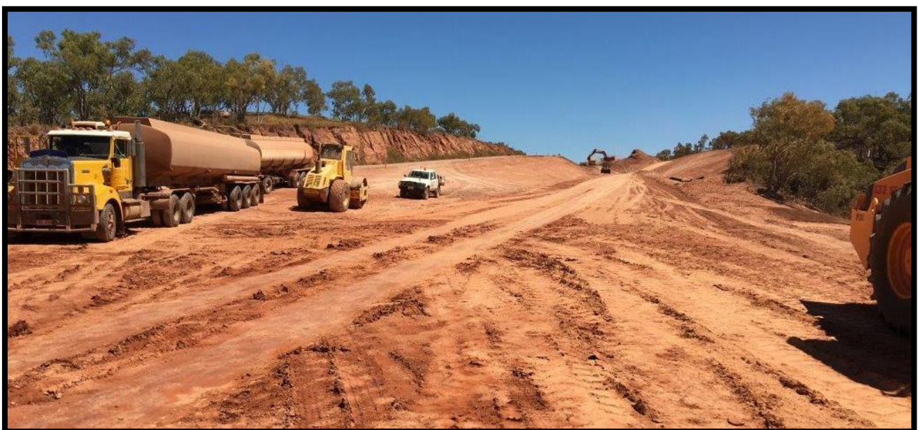
Construction Photo: Carpentaria Highway – pavement strengthening and widening Borroloola Jump Up chainage 229.0 - chainage 233 km
