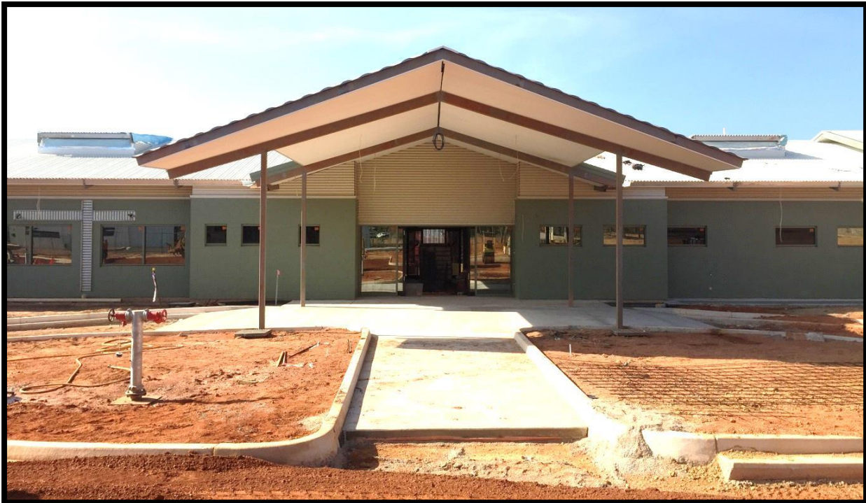
Construction Photo: Nhulunbuy High School - residential boarding facilities - stage 1 - 40 bed residential facility and ancillary infrastructure
