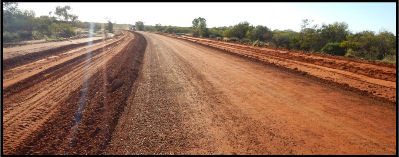
Photos: Sandover Highway - gravel re-sheet approximately 9 kilometres between chainage 227 km and 236 km
