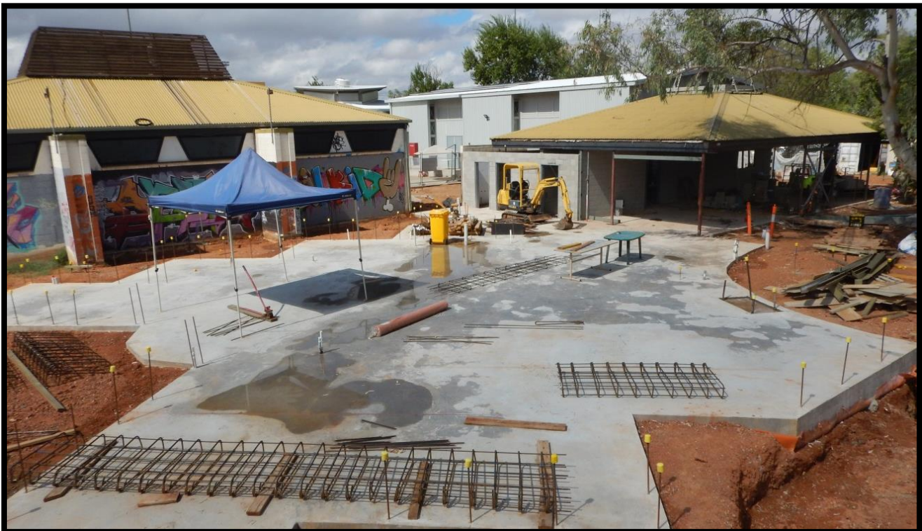
Photo: Alice Springs - Wills Terrace - Youth and Community Centre - upgrade existing and construct new Wellbeing Centre
