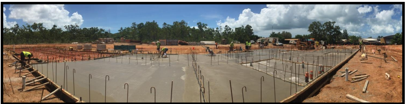
Photo: Nhulunbuy High School – new boarding facility – administration building slab - under construction
