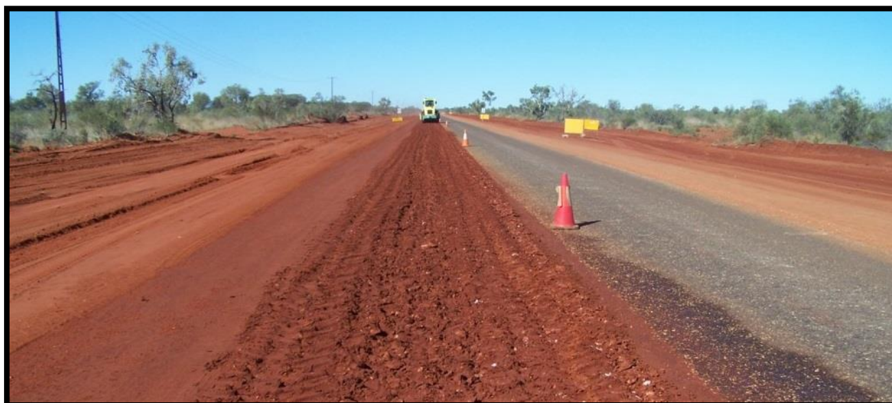
Construction Photo: Alekarenge - Kinjurra Road (Ali Curung Access Road) shoulder upgrade and reseal
