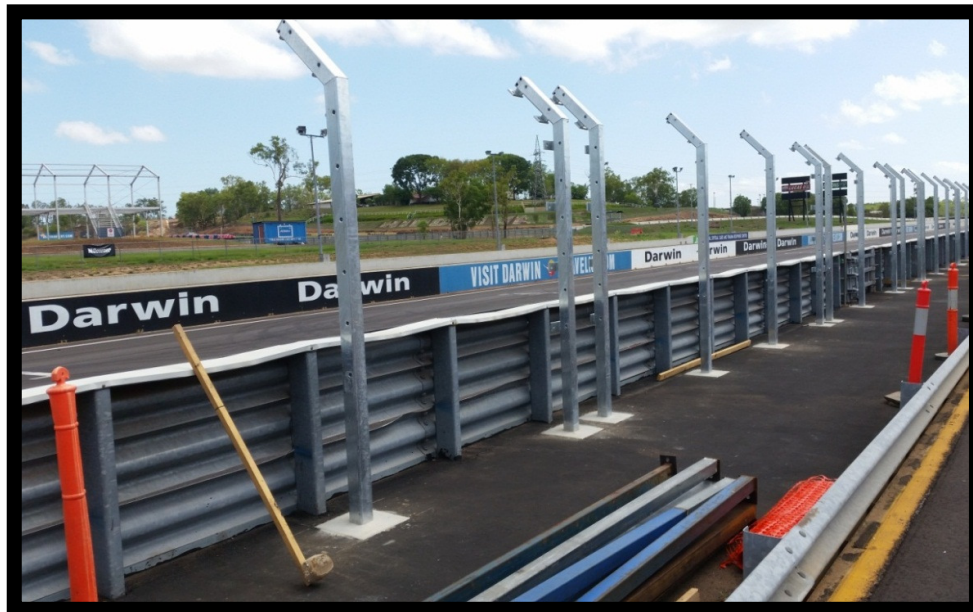
Photo: Poles installed for the debris barrier on the main straight at Hidden Valley Motor Sports Complex
