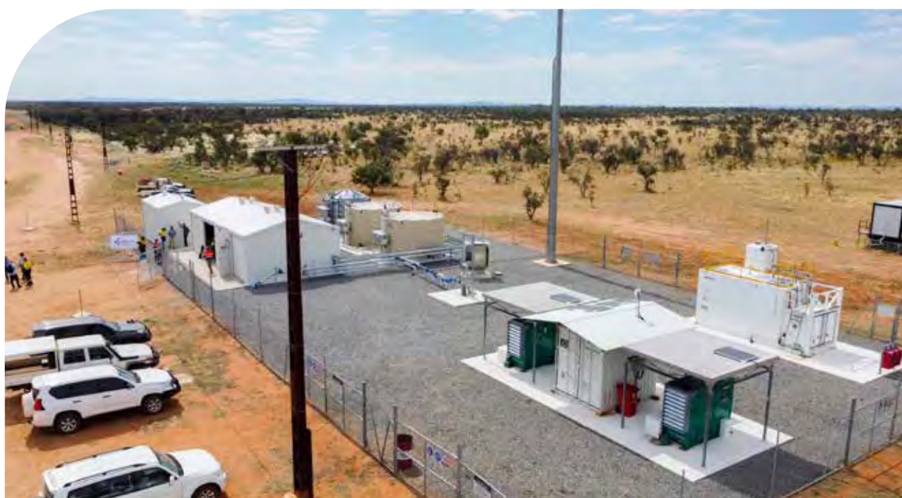
Above: Laramba Water Treatment Plan. Credit: Territory Families, Housing and Communities.
