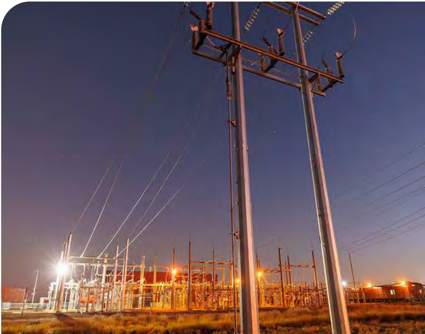
Above: Owen Springs switchyard, Alice Springs. Credit: Power and Water Corporation.
