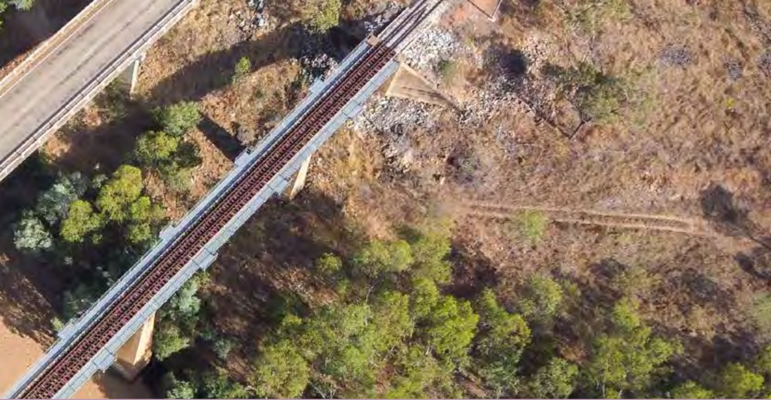
Left/above: Stuart Highway bridge and railway crossing. Credit: Territory Families, Housing and Communities Central Australia.
