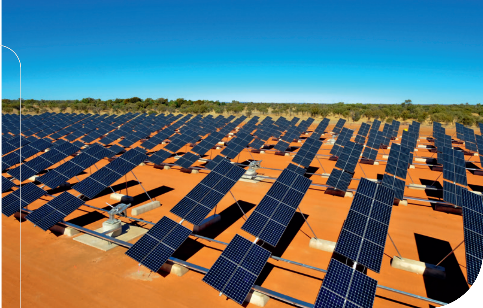
Above: Uterne Solar Power Station, Alice Springs.
