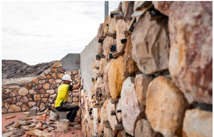
Above: A JT Harvey Construction worker erects stone cladding on the ramp to the new pontoon using the local porcellanite rock excavated from the site during early construction works.
