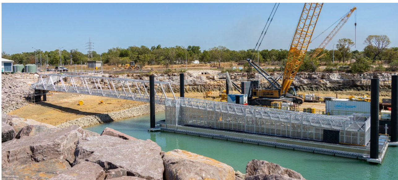
Above: The new 34 metre by 10 metre wide floating pontoon and gangways are installed in the new basin.
