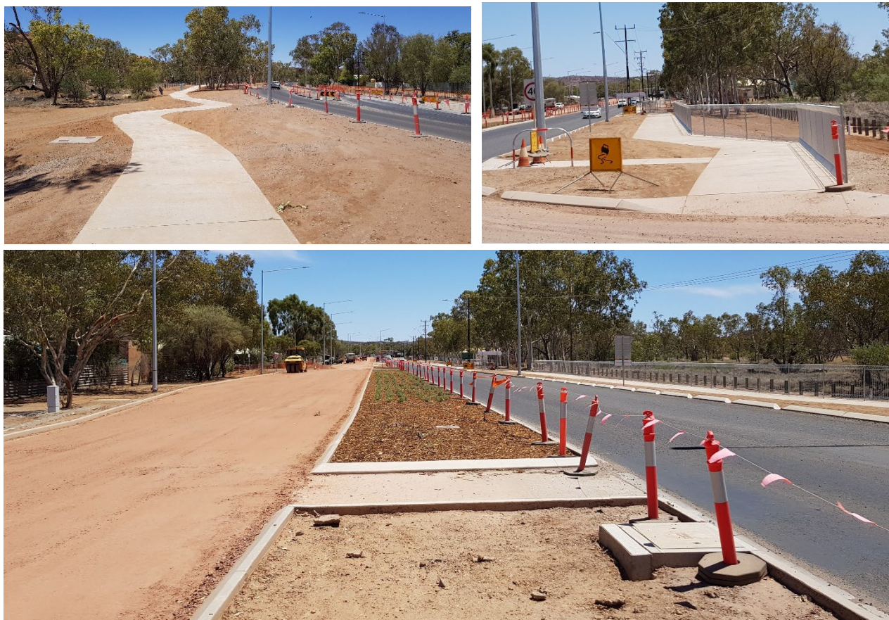
Construction photos: Stuart Highway - upgrades from Motor Vehicle Registry to Herbert Heritage Drive
