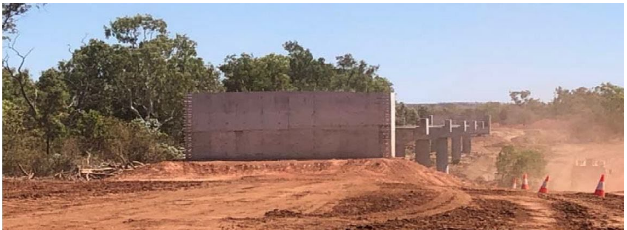
Construction photo: Keep River Plains Road - upgrade stage 1 chainage 0 km to 13.475km
