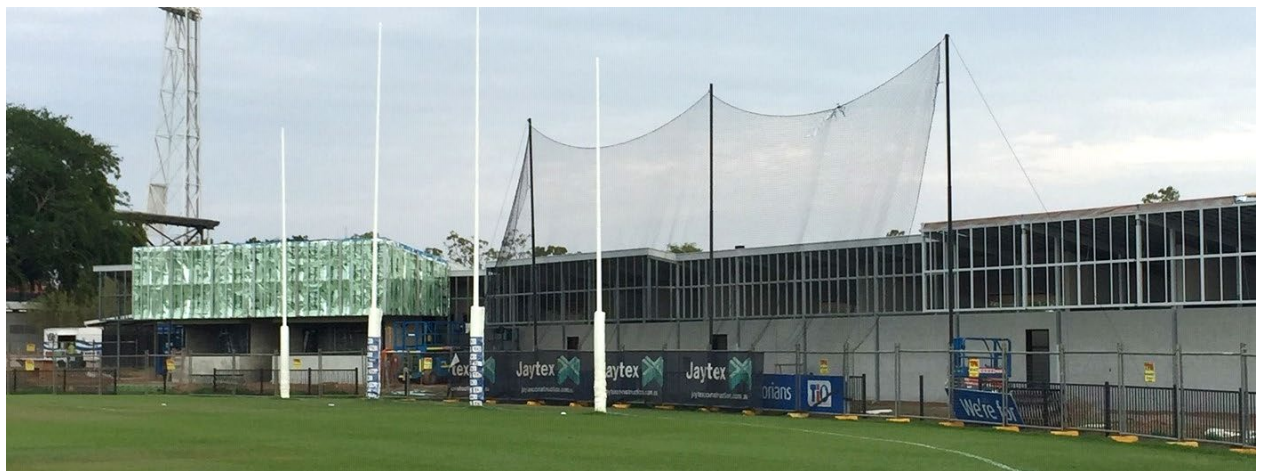
Construction photo: Marrara Sporting Precinct - TIO Stadium field 2 - design and construct new facilities including change room, media room and kiosk
