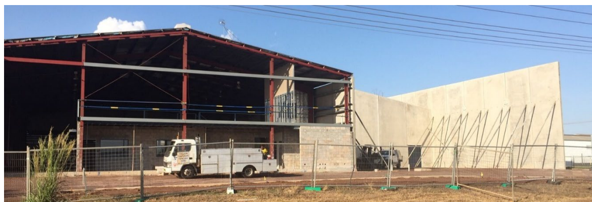
Construction photo: Pinelands - 892 Stuart Highway - extensions to existing warehouse, showroom sales and offices
