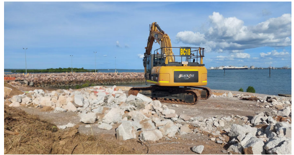
Above and far below: Local business Black Cat Civil starts work on the ship lift facility site to demolish existing concrete structures.
