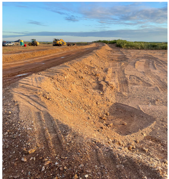
Below: Work is completed to prepare ponds at East Arm for dredge spoil placement.
