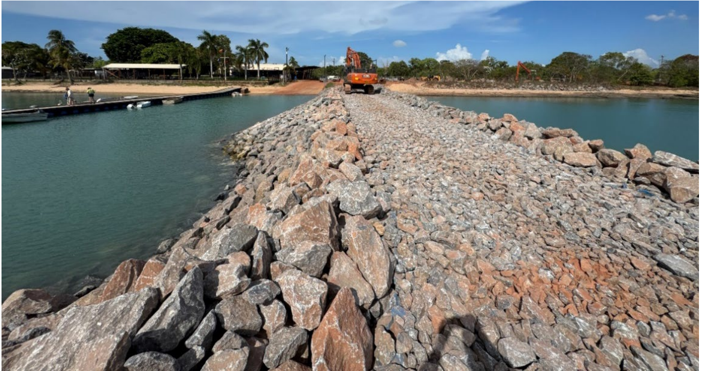
Above: Work progressing to build the rock groyne at Gove Boat Club.
