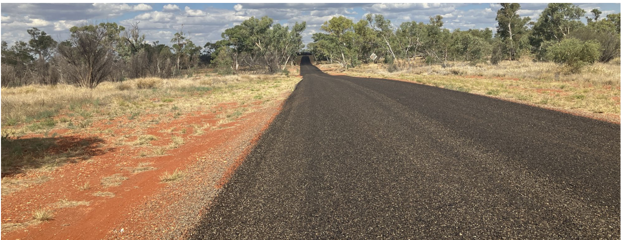
Engawala Road - flood damage reinstatement
