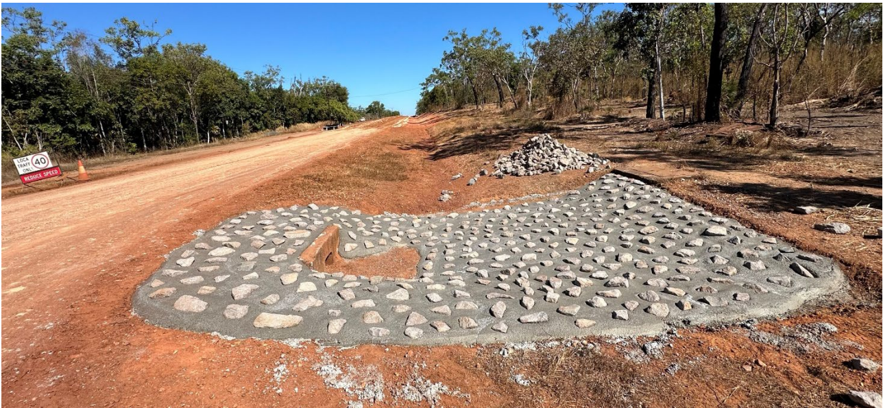
Guys Creek Road - upgrade gravel to seal. Images courtesy of Litchfield Council and Colemans Contracting and Civil
