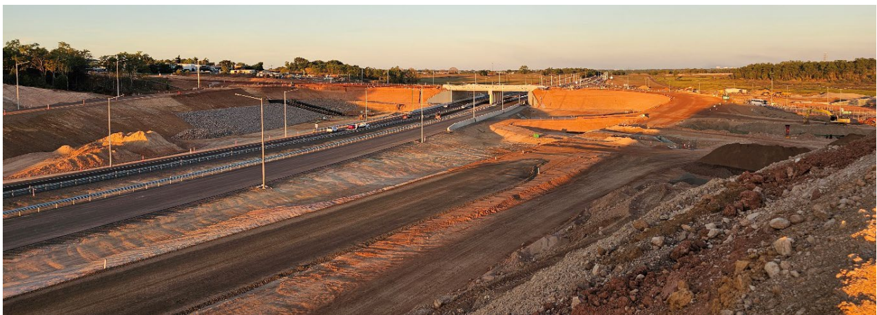
Tiger Brennan Drive - design and construct overpass at Berrimah Road intersection. Photos courtesy of Sitzler
