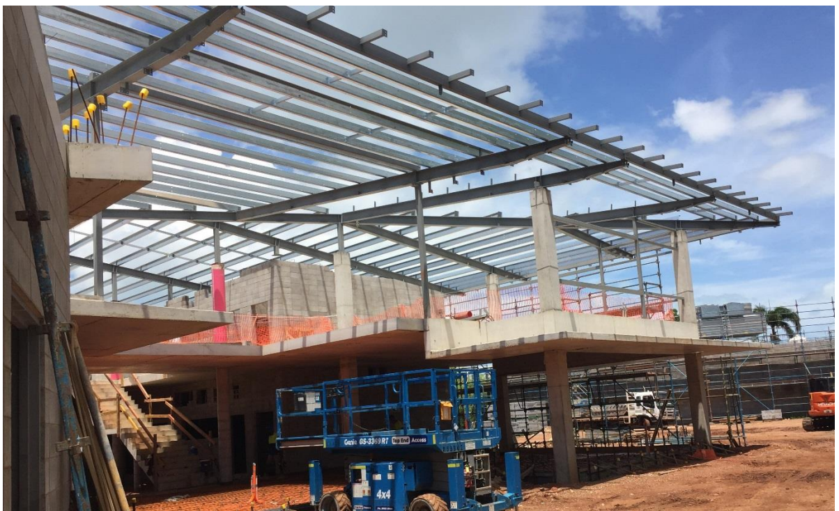
Construction photos: Darwin High School - new Science, Technology, Engineering, the Arts and Mathematics (STEAM)
