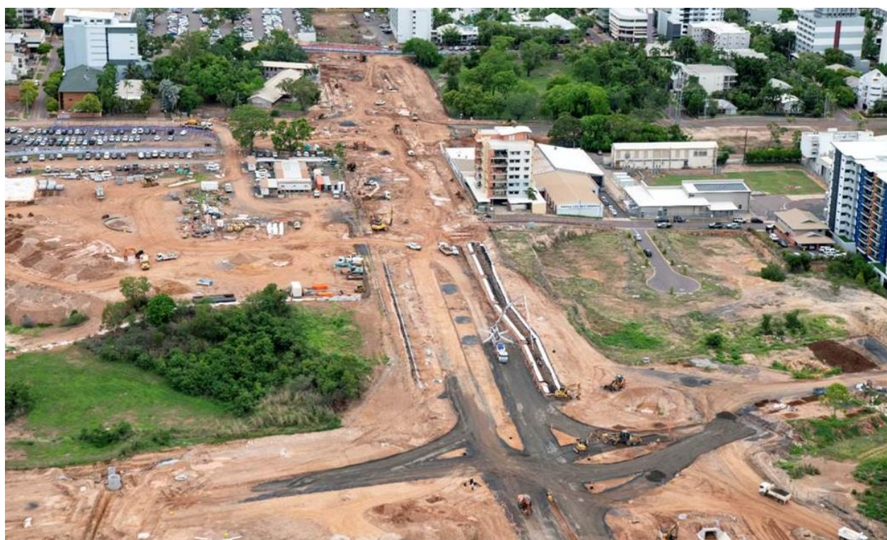
Construction photo: Darwin CBD - Garramilla Boulevard Link - duplication of Tiger Brennan Drive from Dinah Beach to McMinn Street (stage 3)
