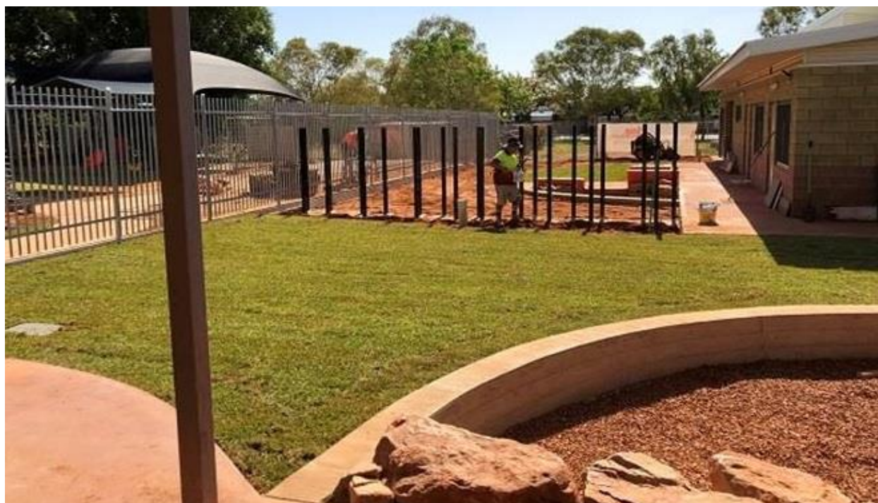
Construction photos: Tennant Creek Early Childhood Integrated Learning Hub - new preschool & child & family centre
