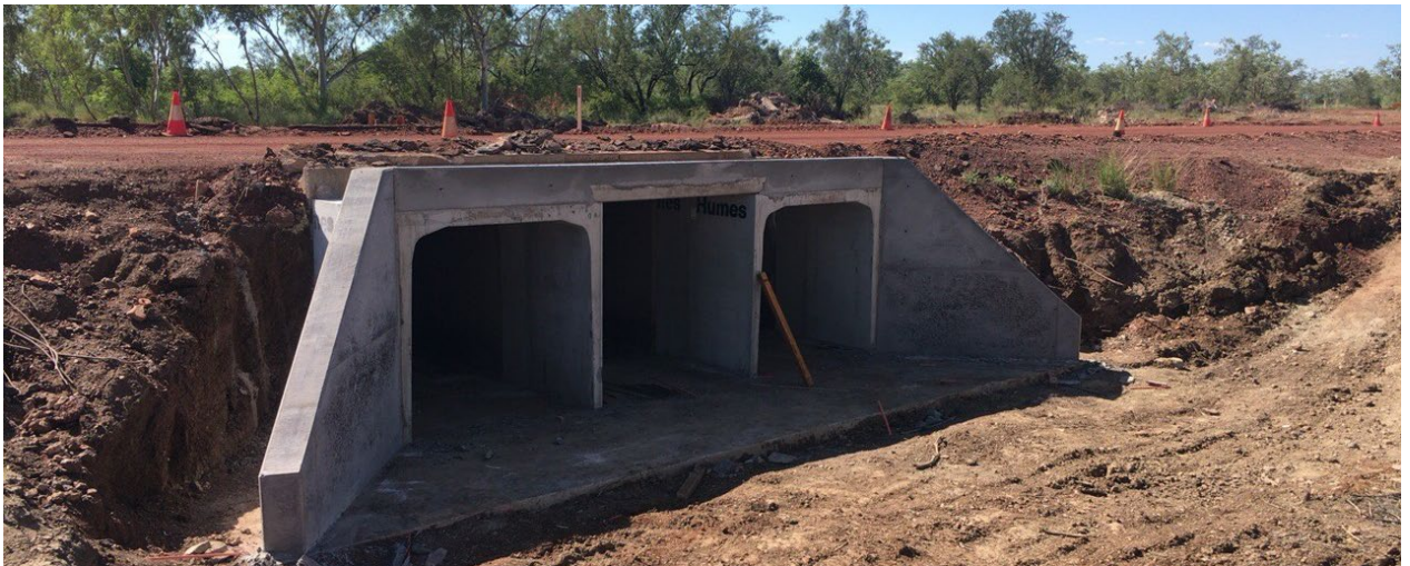
Construction photos: Tablelands Highway - supply, delivery and installation of culvert structures and upgrade existing road between chainages 303 - 318 km
