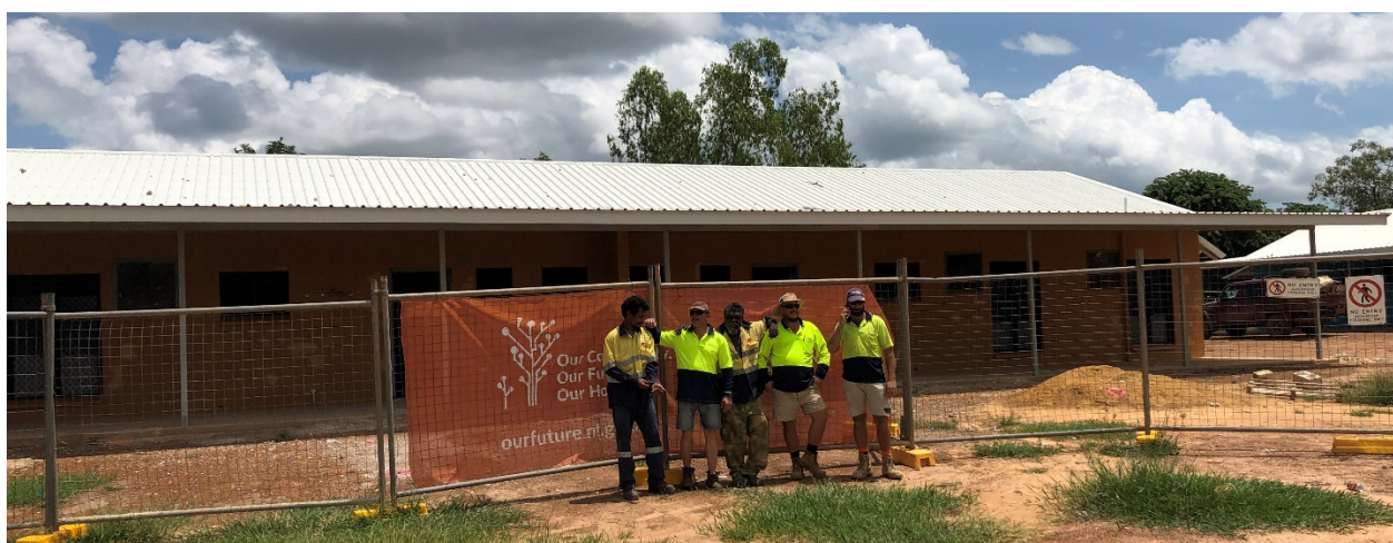
Construction photo: Nganmariyanga - HomeBuild NT - construct 4 by 3 bedroom and 1 by 4 bedroom dwellings
