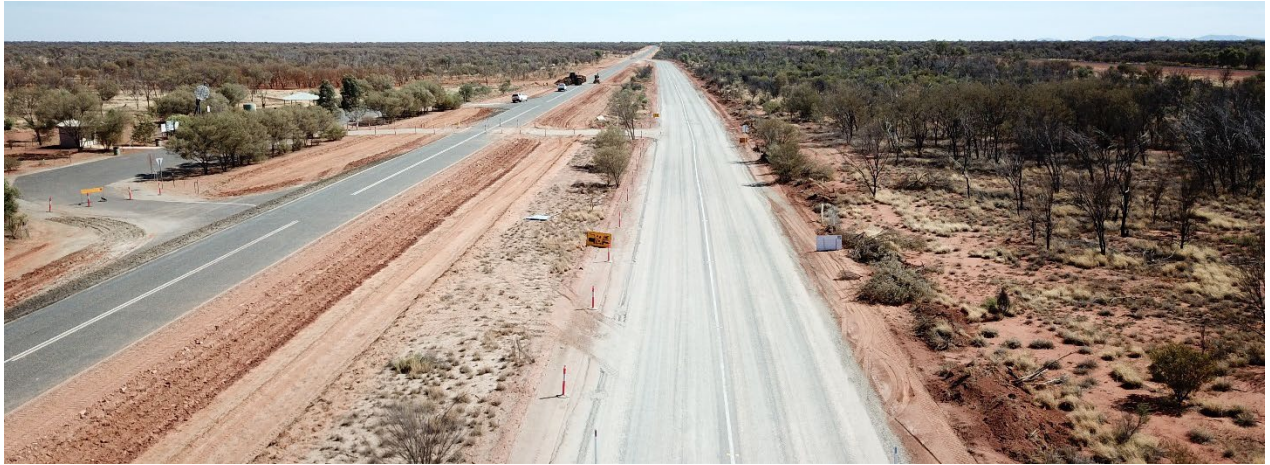
Construction photo: Stuart Highway - upgrade access to Tropic of Capricorn rest area
