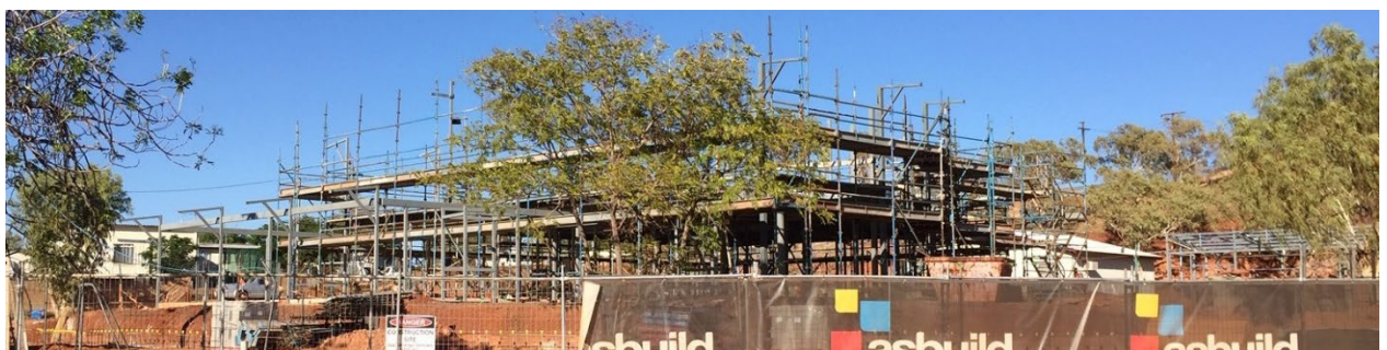
Construction photo: Tennant Creek - Irvine Street - Anyinginyi Health Aboriginal Corporation - new office building, associated structures and car parking
