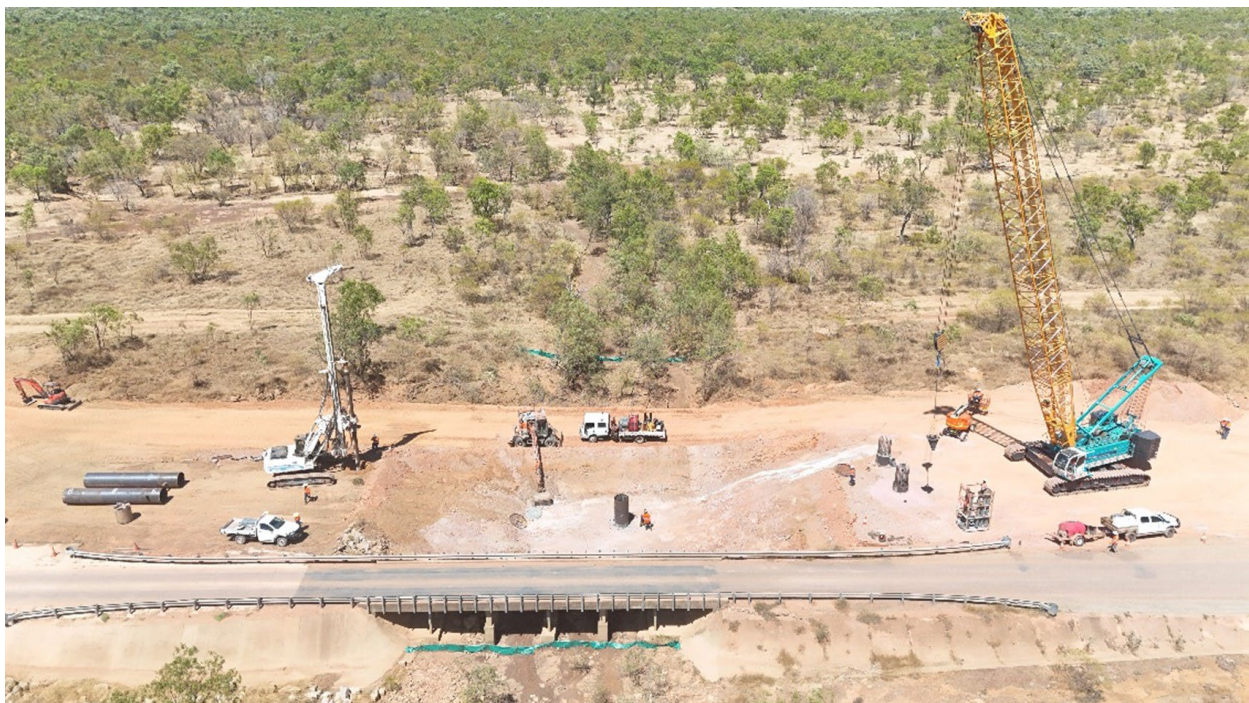
Carpentaria Highway - design and construct upgrade to 2 lane seal - 140 - 175 km including demolish and construct October Creek Bridge. Photo credit: Exact Construction
