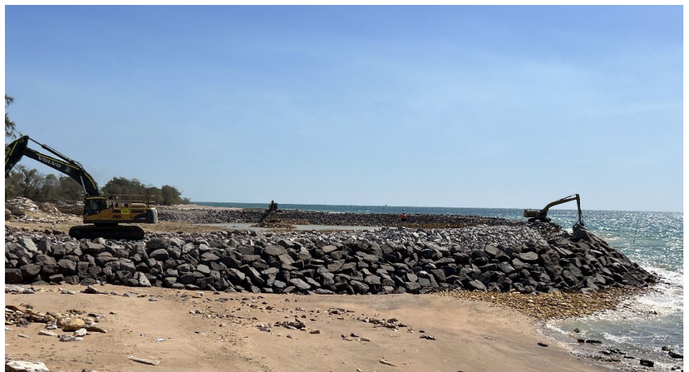
Construction of the southern and northern breakwaters continues on site for the Mandorah Marine Facilities project.
