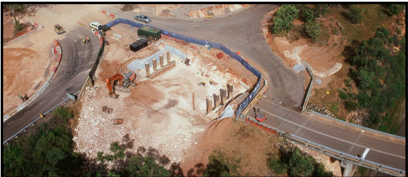
Photo: Tiger Brennan Drive – works commence on new bridge at Hidden Valley
