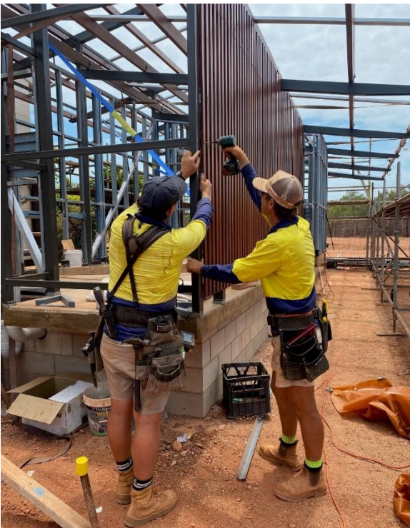
Deltareef employees Mitchell Street and Klay Mercer put up the milled Stringybark Eucalyptus timber as part of a new amenities building at the Gunyangara Tourism Precinct project.
