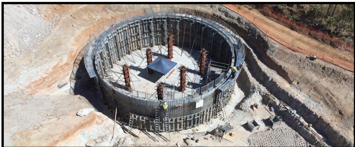
Photo: Palmerston East - Zuccoli west sewer pump station and rising main
