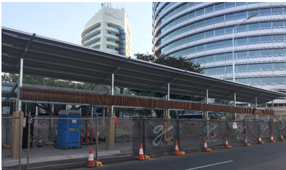
Construction photo: Darwin CBD - Bennett and Smith Street - design, document and construct covered walkways
