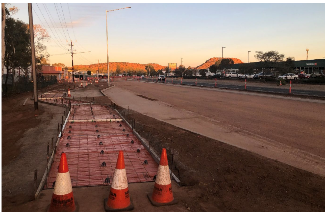
Construction photo: Stuart Highway - upgrades from Motor Vehicle Registry to Herbert Heritage Drive
