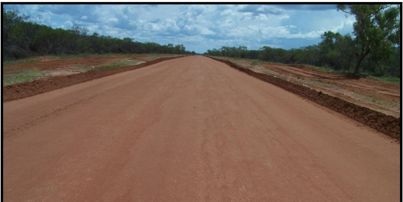
Photos: Tablelands Highway - strengthening and widening the existing pavement sections from chainage 40-43 km
